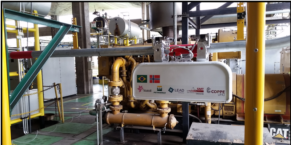
Figure 3.7: DORIS near two red markers installed on the rail base area.
