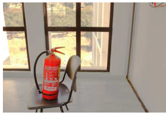
(b) Fire Extinguisher.
