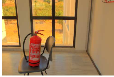
(b) Fire Extinguisher.
