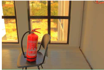
(b) Fire Extinguisher.
