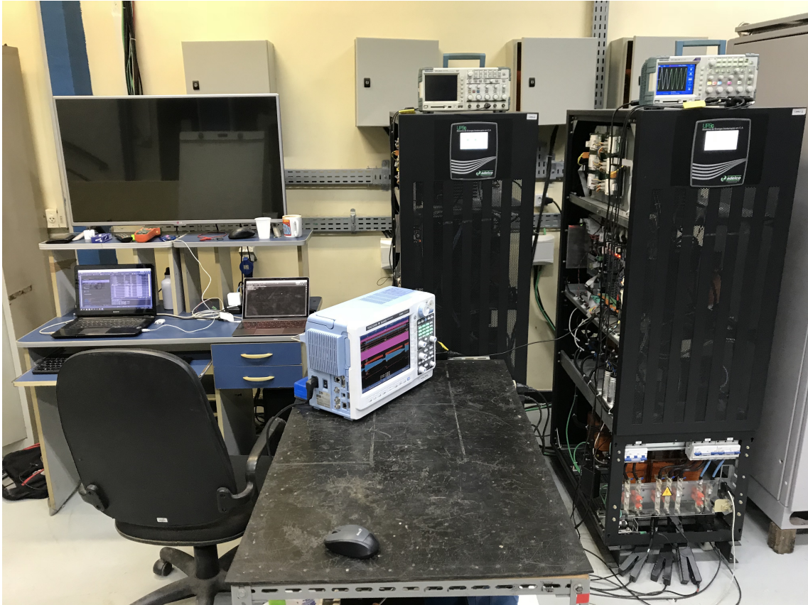
Figure 5.15: Test rig composed of two back-to-back converters connected in parallel. Also in the picture are the computers used for embedded code loading, debugging and supervision, and the oscilloscope used for all shown measurements, a Yokogawa DL850EV .
